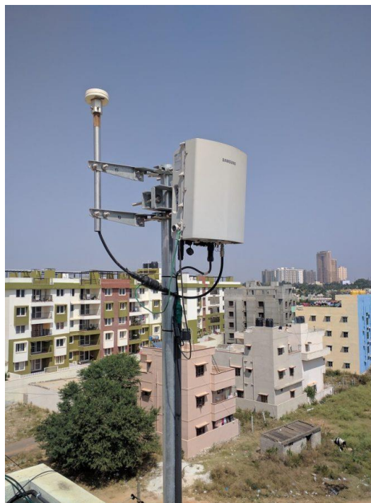
Figure 19: A 5G small cell signal router
